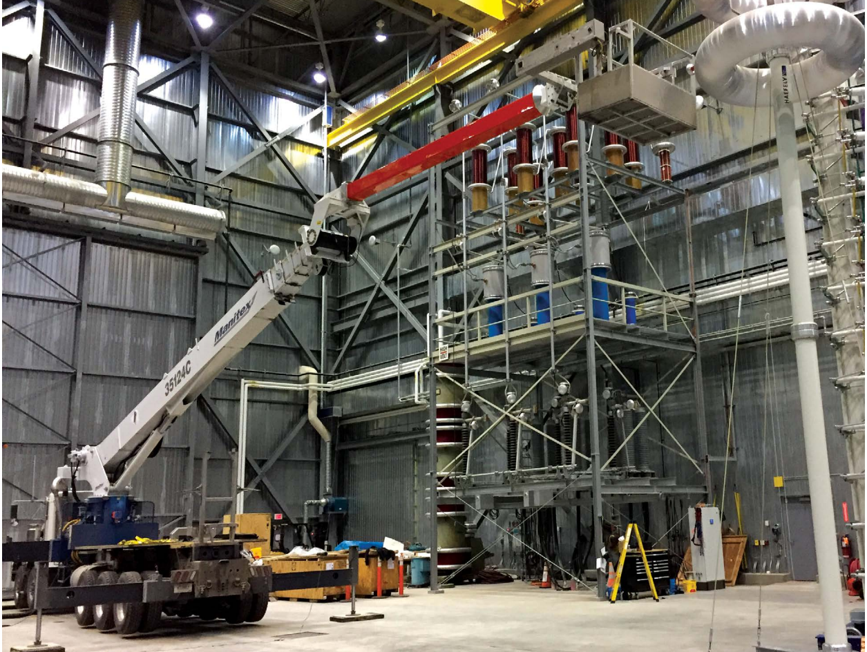
2,400 kV lightning impulse generator performing switching.
